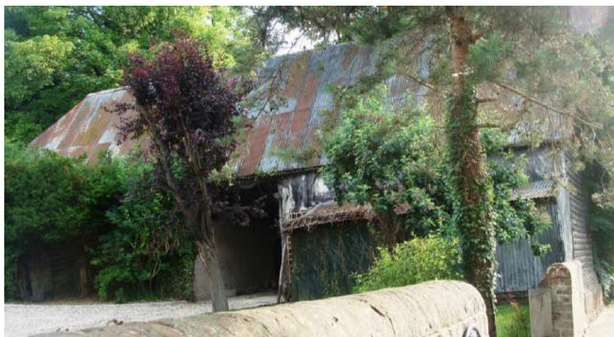
Picture 45. Grade II barn at Little Meadow, the corrugated roof was originally thatch. A thatch replacement roof would represent a significant gain. Potential grant assistance may be available. The building is on the Council's Heritage at Risk Register.
