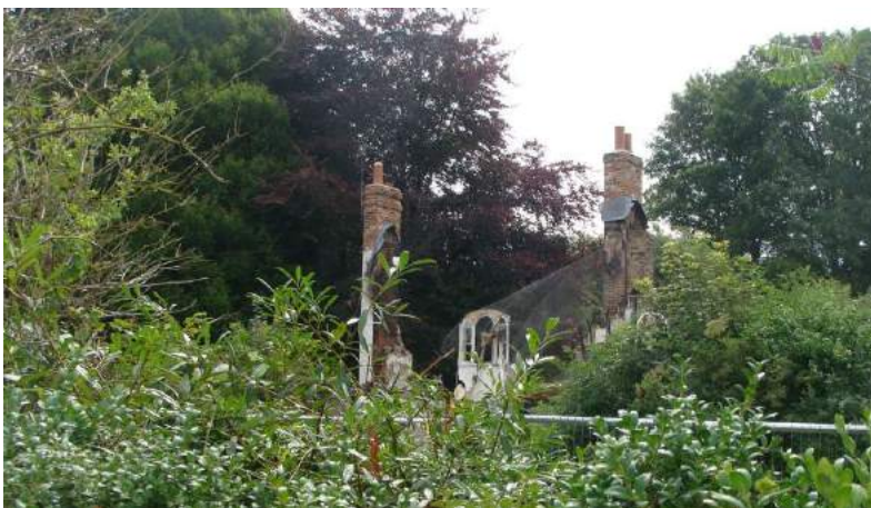
Picture 34. Hormead Cottage severely damaged by fire (December 2016). Discussions are taking place regarding its restoration.
