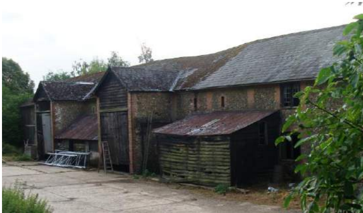
Picture 67. Interesting range of mid/late 19th century barns now to be residential conversion.
